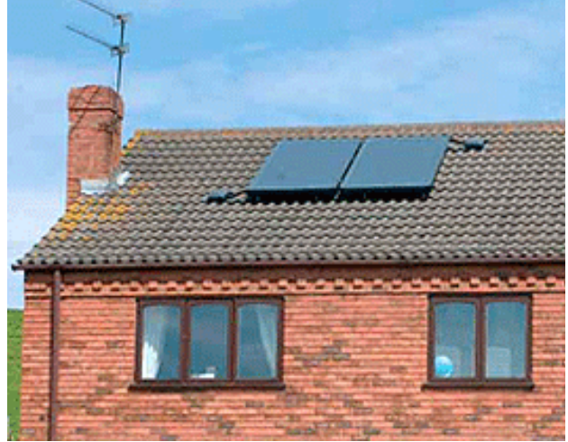
Solar heating system...
